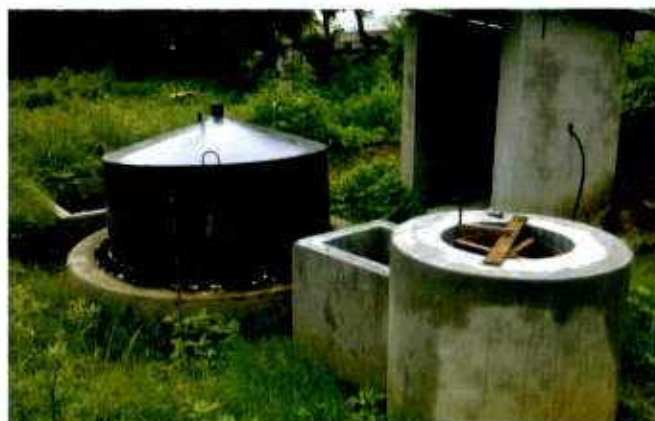
Figure 1: Bio-gas plant installed at CSIR-IIP.
