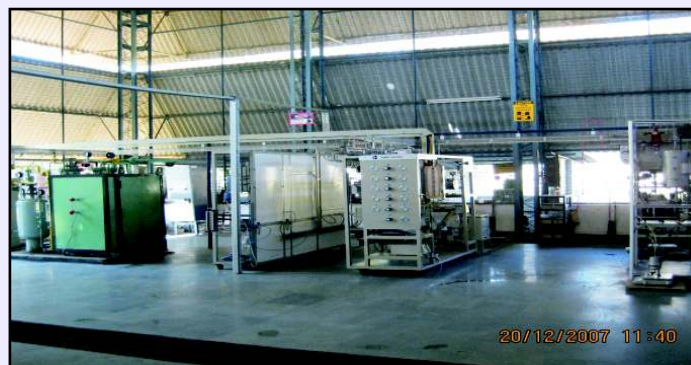
Overview of GTL lab containing Synthesis gas generation unit, high-temperature fixed-bed reactor and high-pressure fixed-bed reactor units for FT and DME synthesis
