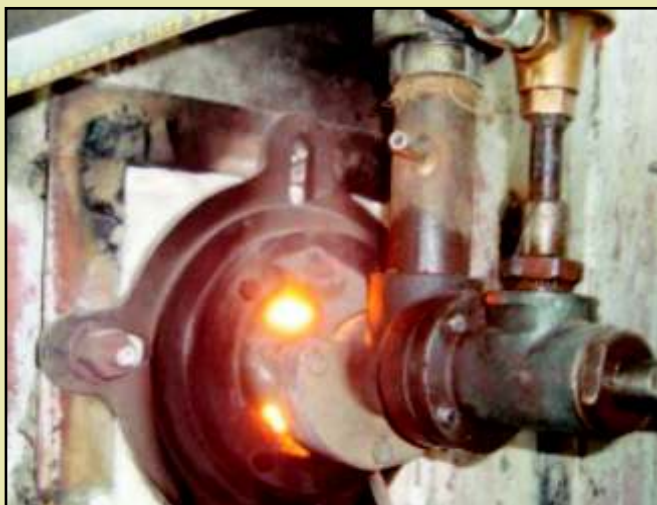
IIP LAP burner during operation on tunnel kiln
